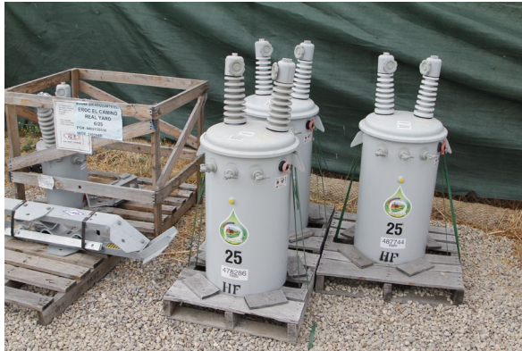
SINGLE PHASE OH TRANSFORMERS
