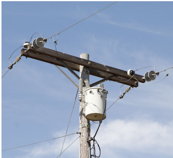
SINGLE PHASE OH TRANSFORMER
